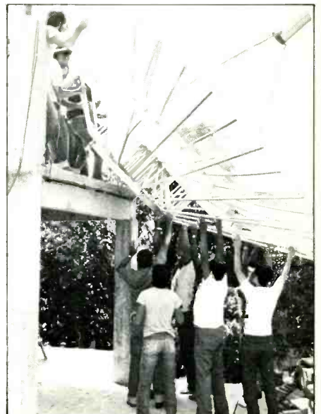
Relocation at a 5 meter satellite earth station is no problem with a crew this large!
